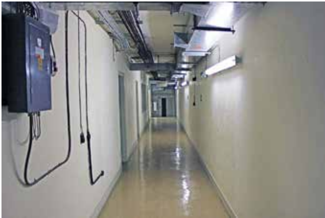
View of lower level corridor showing exposed ventilation and electrical services
